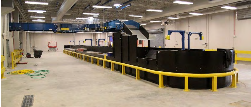
The Eastern Iowa Airport passenger terminal airline baggage area Photograph by Mead & Hunt, Inc. (2011)
