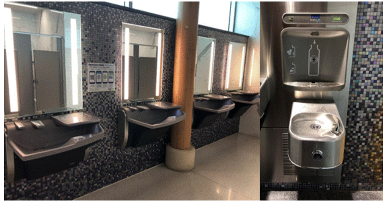
Figure 1.18: Water Efficient Fixtures
